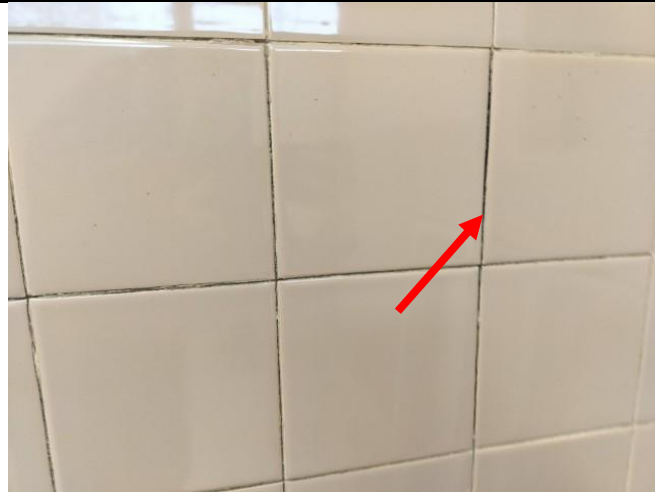
Photo 9: View of the visual suspect mould growth (see arrow) observed on the non-asbestos containing ceramic tile grout on the wall within the Boy's Washroom.
