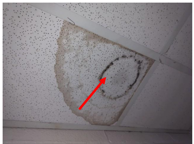
Photo 12: View of the visual suspect mould growth (see arrow) observed on the non-asbestos containing acoustic ceiling tile outside of the Gymnasium Door.
