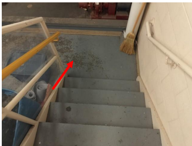
Photo 8: View of the low-level lead containing grey paint (see arrow) observed to be in fair condition on the floor of the Mechanical Room.
